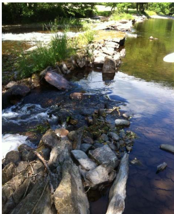
Photo 2: Dulverton Weir section showing flat facing stones (now buried under the temporary repair).
